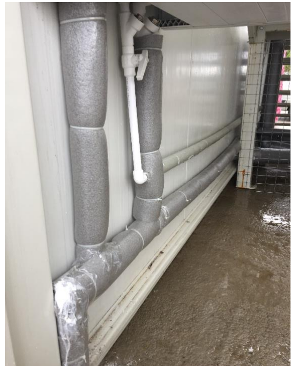
-Pipes Outgoing from the Outer walls of the container
