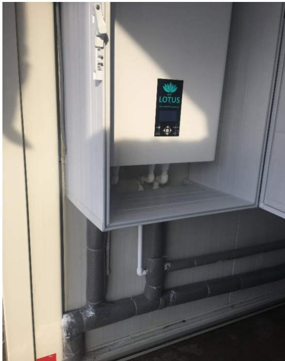
-Combi Boiler View
